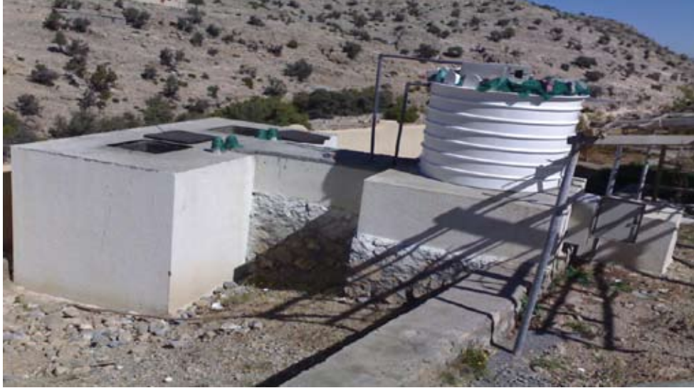
The constructed treatment system in Al Jabal Al Akhdar, Oman
