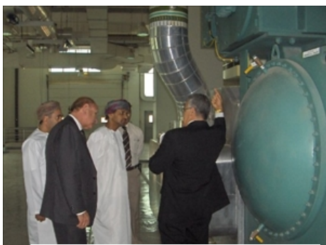
Figure 15--District cooling systems can provide substantial energy savings.
